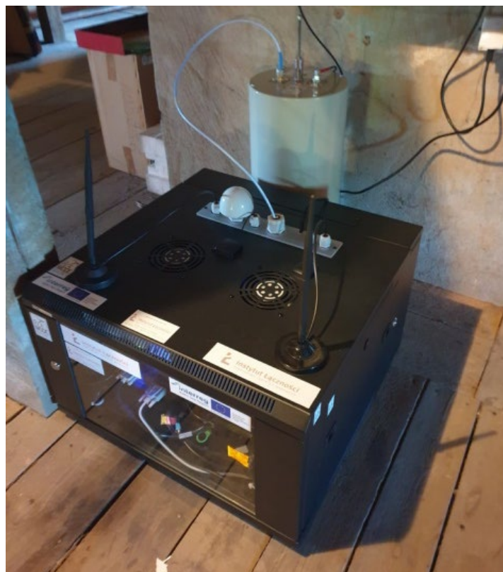
Figure 3-1: Receiving station in Jastarnia
